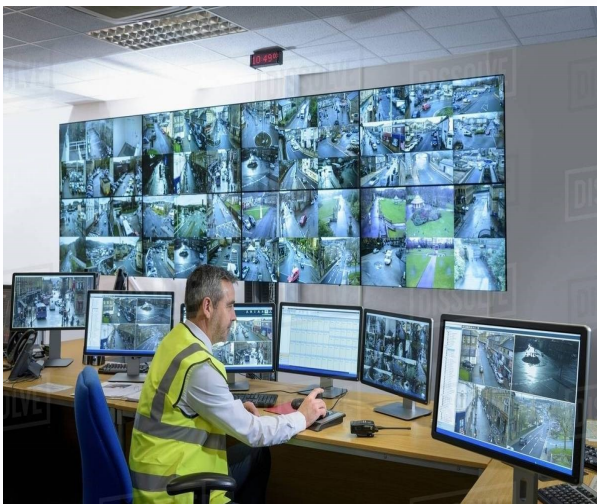
Security Control Systems
