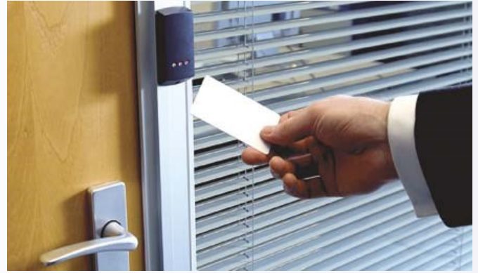
Door access Control Systems
