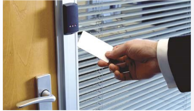
Door access Control Systems
